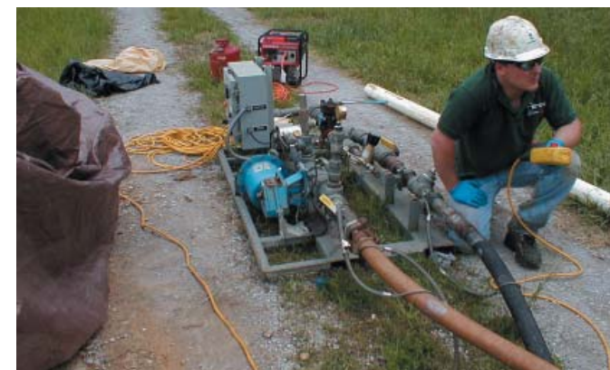
An ARS Engineer Operating one of our Gas Injection Modules.
